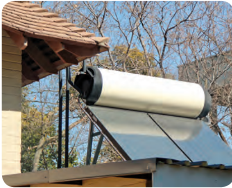
Solar water heater at Peech Hotel
