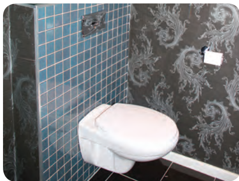
Water efficient dual-flush toilets at the Peech Hotel
